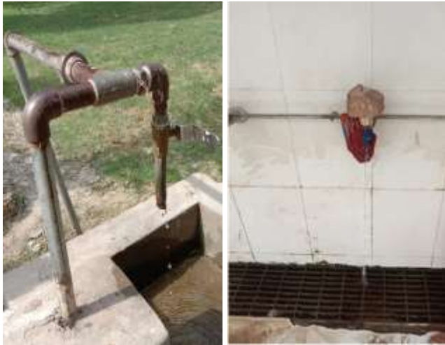
Fig. 2. Site observations for Malfunctioned Water Tap
