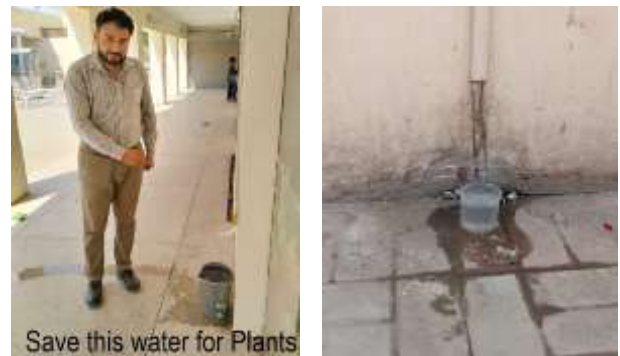
Fig. 4. Site observations for AC water Collection.
