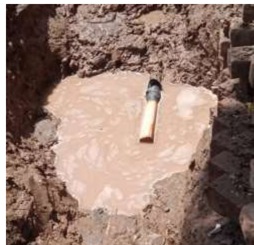
Fig. 1. Site observations for Underground Piping system leakages
