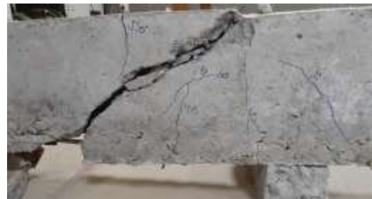
Flexure Cracking of Beam at 30° Angle
