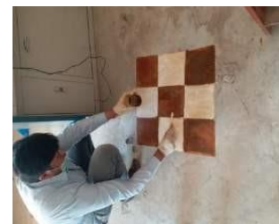
Applying iron sulfate and copper sulfate acid stain to the laboratory floor at BZU (Bahauddin Zakariya University) Multan
