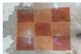
Acid-stained area washed after ammonia solution application
